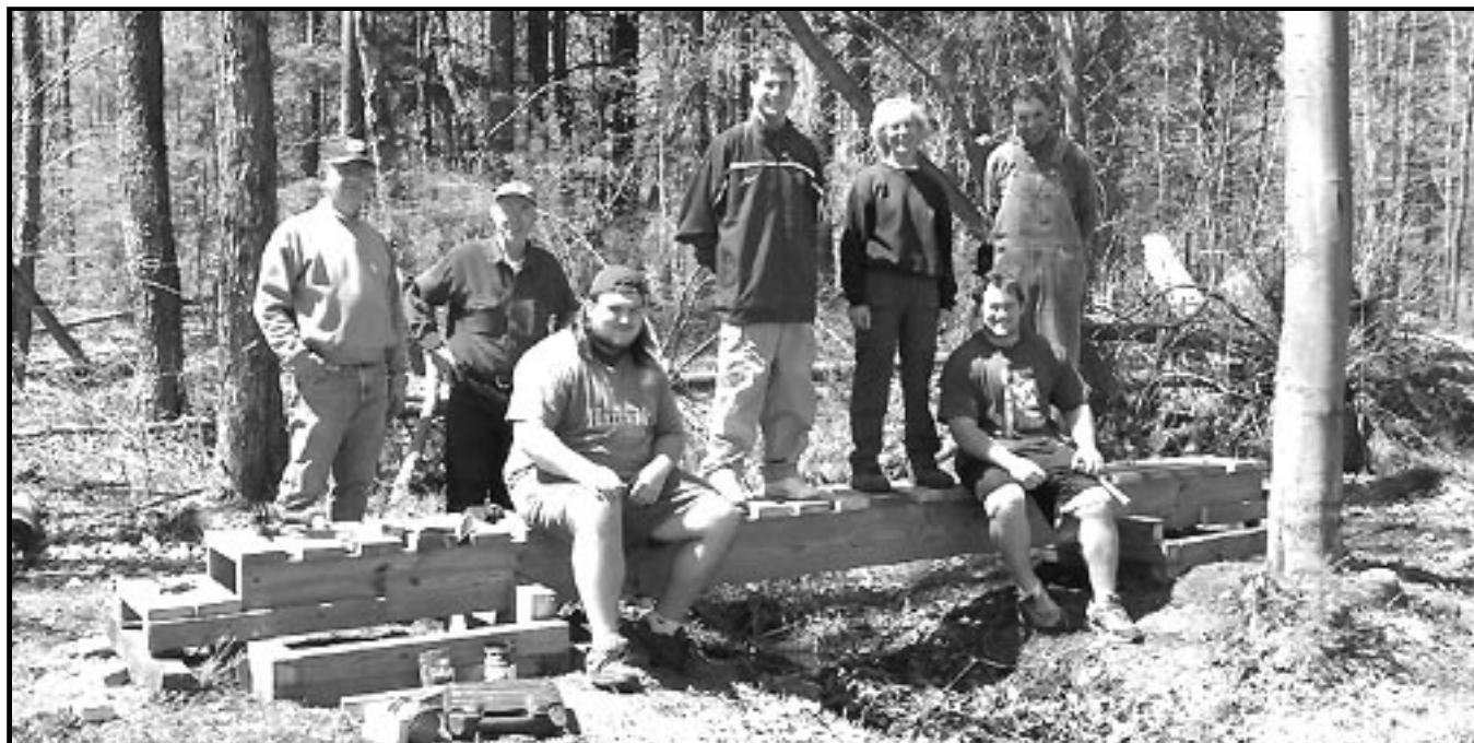
Susquehanna Chapter members and Hartwick College volunteers with our newly-constructed bridge in Arnold Lake State Forest, May 7, 2005. Photo by Danny Birnbaum
